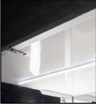
Illuminazione a led LED lighting
